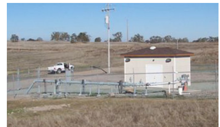
Above, "Well 14" on the Lake Camanche Village water system. Well 14 was constructed in 2008 to assist in meeting water needs as other Camanche system wells declined in yield.
