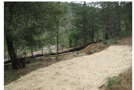
Above, Tree removal and erosion control at Gayla Manor in preparation for expanding the subdivision's current over-taxed leach field. Work on the leach field itself will begin once the rainy season is over.
