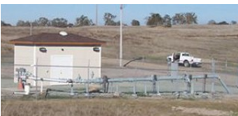
Lake Camanche's Well 14 needs repair due to water quality problems.
